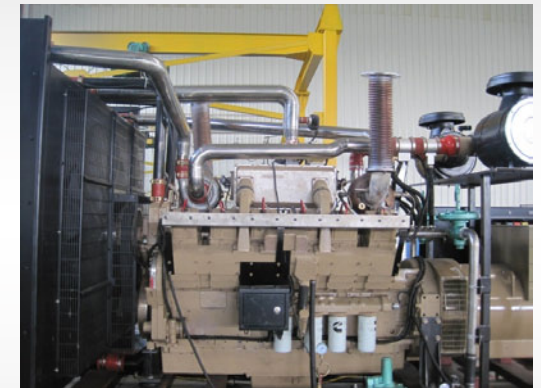
Natural Gas Genset 600kW—Utility Gas
