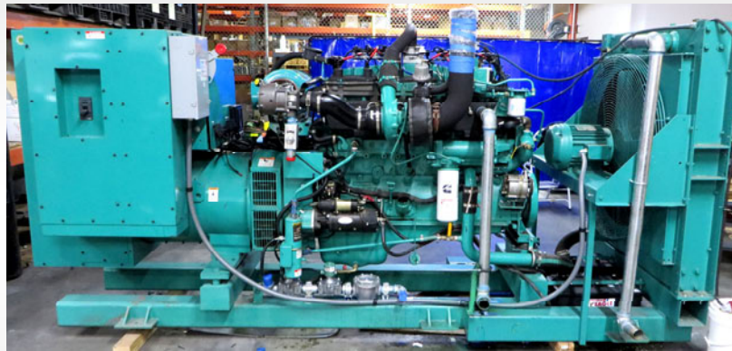
Biogas Genset 230kW—Fruit Waste Digester
