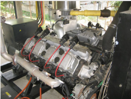
Biogas Genset 125kW—Hog Farm
